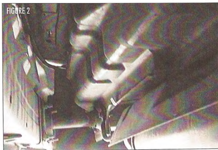
Bumper impact absorbers (the horizontal tube seen here from below, bolted to the bumper at left) are best viewed from the side of the car opposite from the absorber in question.
